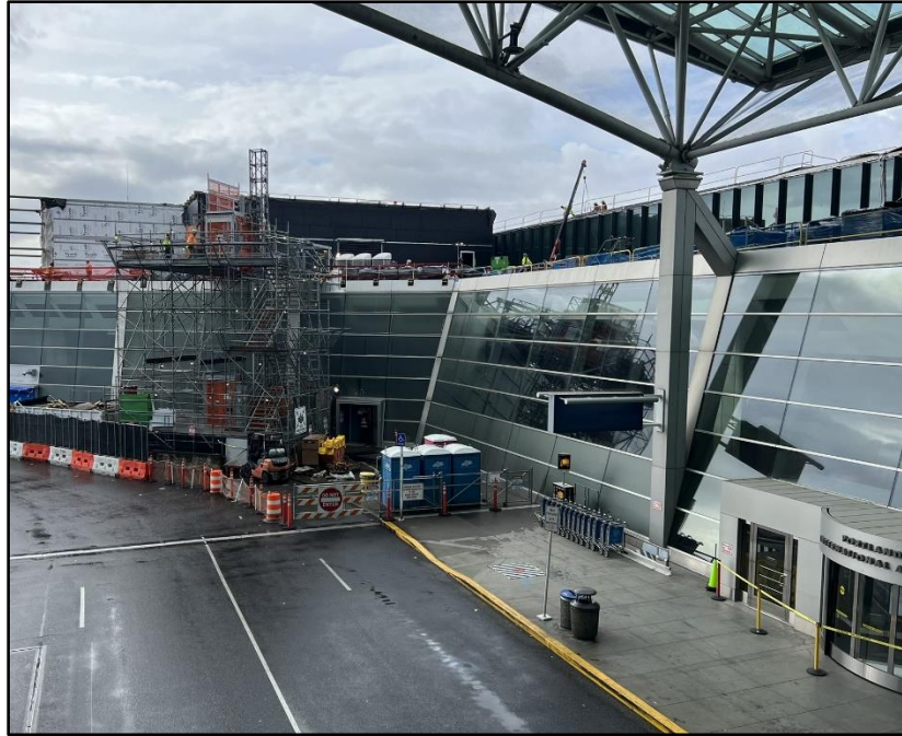
Window curtain wall and revolving door on departures level. These will be replaced on both the arrivals and departures levels in 2026. (Photo: Jeff Broderick)
