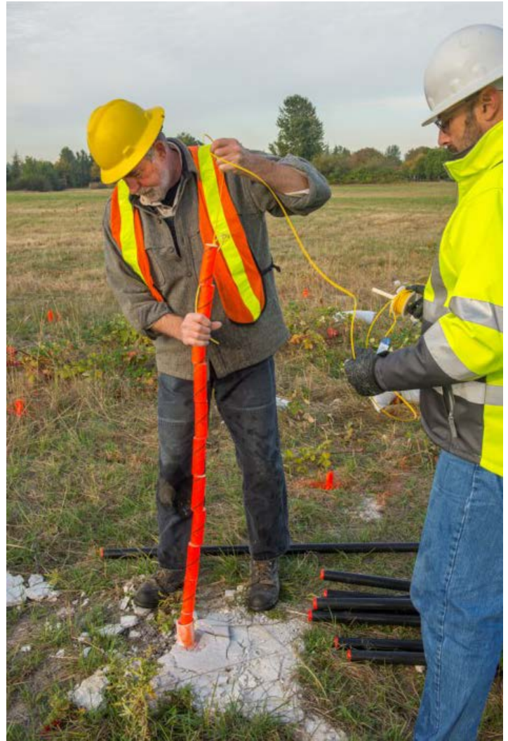
Soil liquefaction testing at PDX, as part of the Port's resiliency planning. Resiliency has been a continued focus of the CAC.
