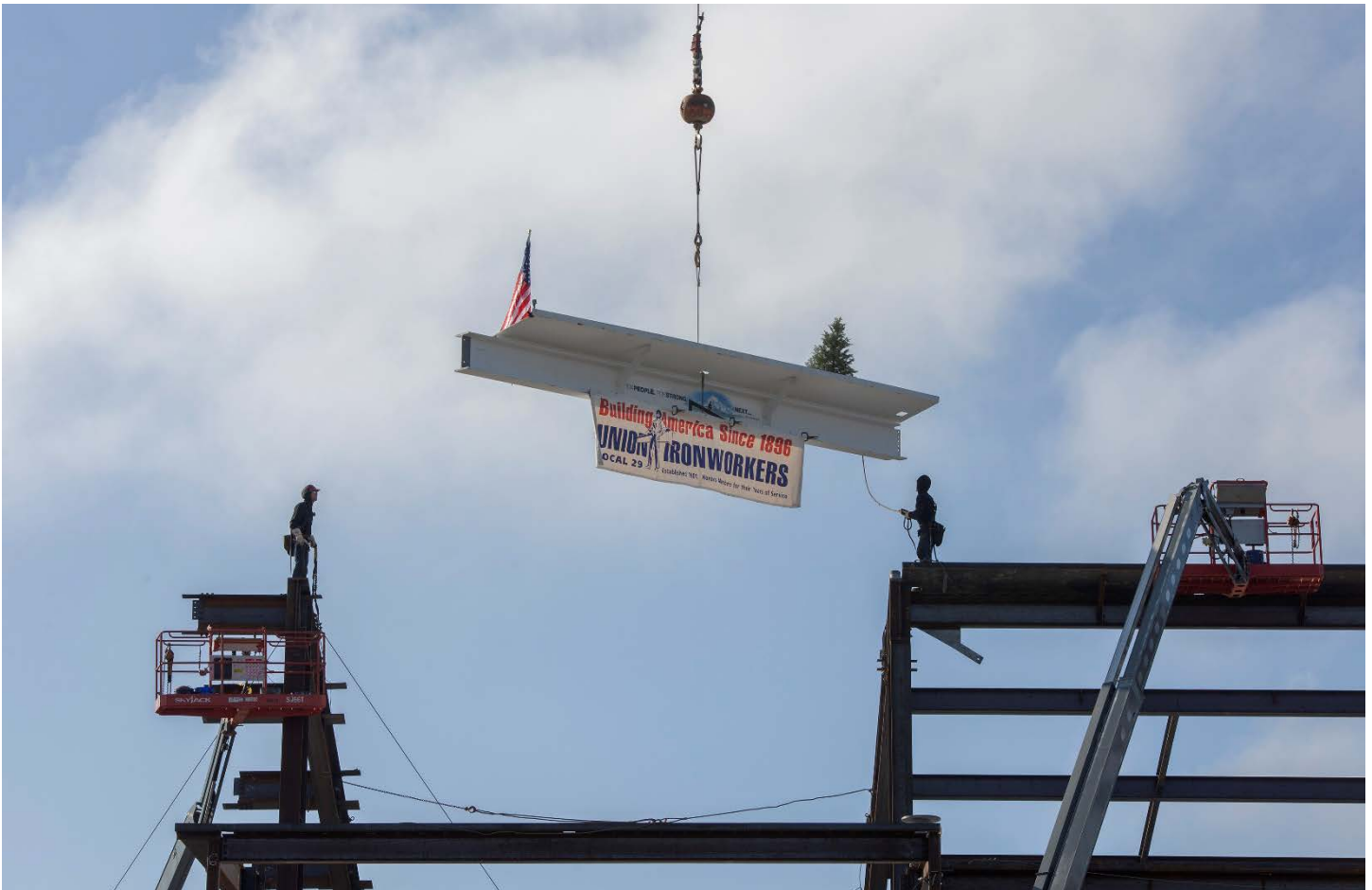
Construction workers install the final beam for the Concourse E expansion, the first major endeavor of the PDX Next Terminal Balancing project. The PDX CAC provided input on this project, which maximizes existing facilities, creates future flexibility and enhances the passenger experience.
