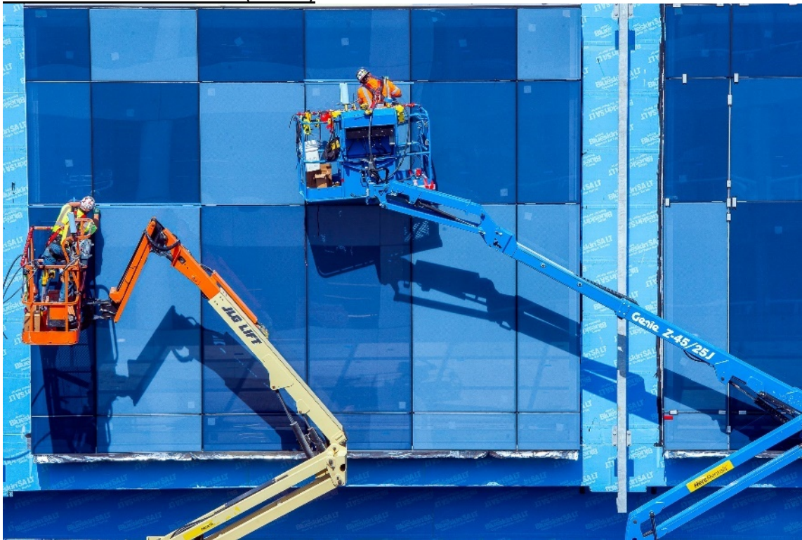
Workers are installing 350,000 pounds of glass to bring you more Pacific Northwest light.
