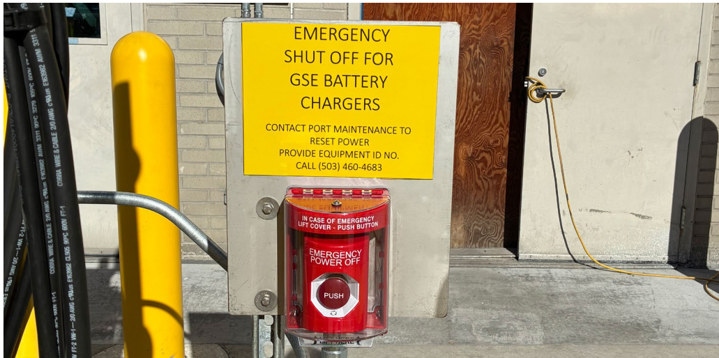
Figure 8: Emergency Shut-Off Button on Charging Stations; Source: Port of Portland.
