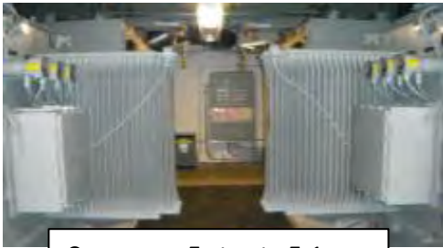
Concourse E at gate E-1 Rm. E1000: TE-A and TE-B
