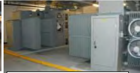
Concourse C, West at Gate C-15, Rm. C1080: TCA and TCB
