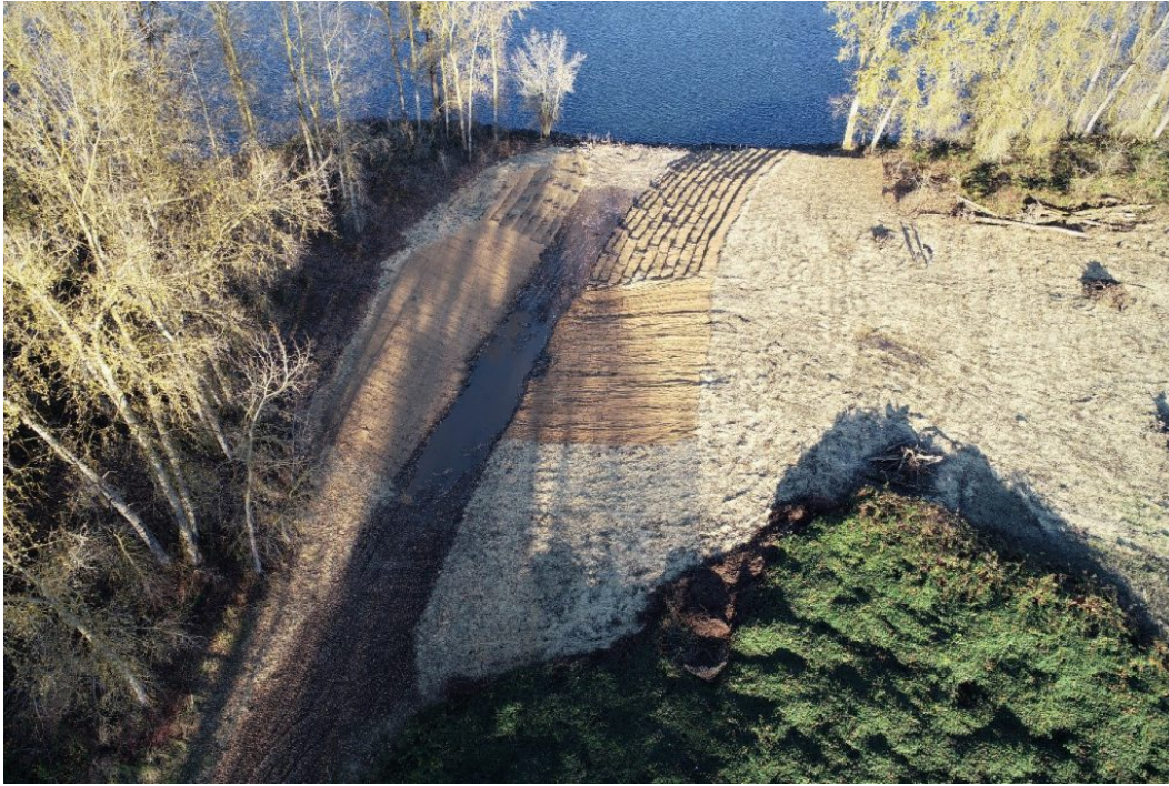
View as of Nov. 2019: Water now flows from the river and toward Jewett Lake on Government Island
