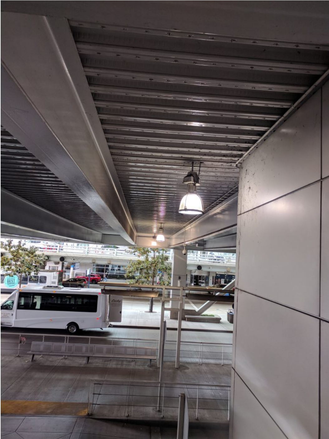
Old Flourescent Fixtures
